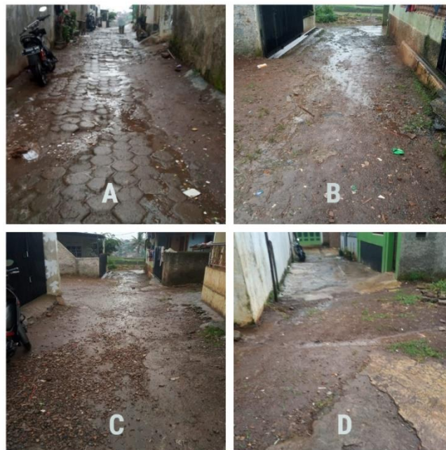
Figure 3. 0% Condition of Environmental Roads RT 01 RW 14 Babakan Cikeruh Village, (A) Upstream Section of the Road, (B and C) Middle Section of the Road, (D) Downstream Section of the Road.
