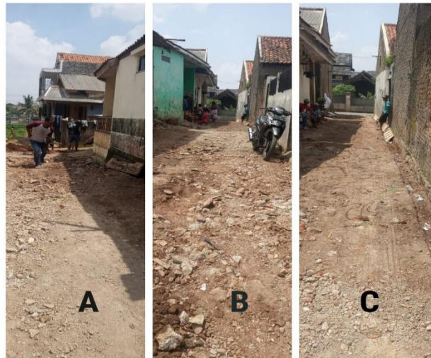
Figure 5. The process of road clearing (A) the results of land clearing on the downstream road, (B) the results of land clearing on the middle road, (C) the results of land clearing on the upstream road.
