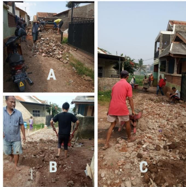
Figure 6. Backfill and Road Leveling Process (A) backfill for middle to downstream roads, (B) backfill for upstream roads, (C) backfill for middle roads (peak point of rainwater diversion)
