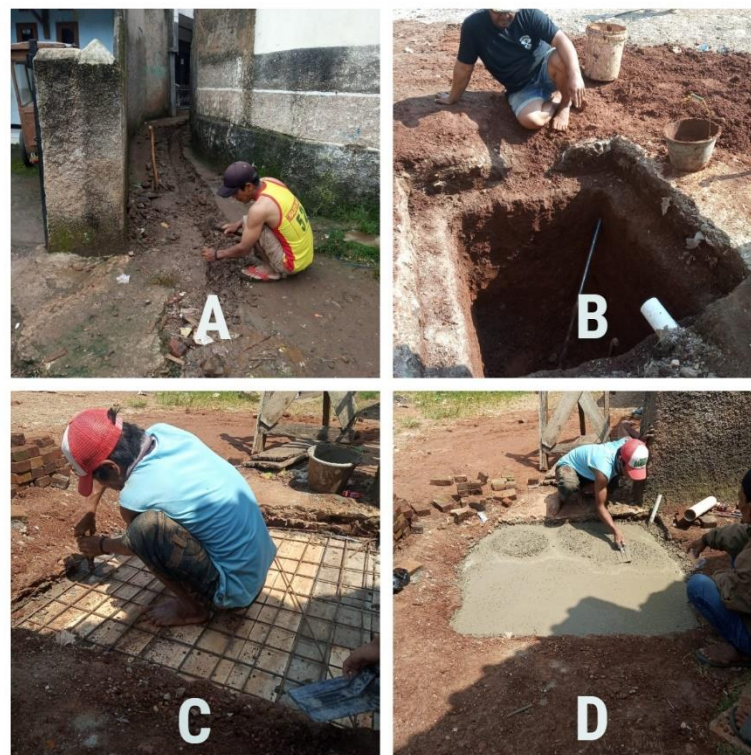
Figure 4. The process of making infiltration wells (A) the process of making sewers, (B) the process of digging infiltration wells, (C) working on ironing infiltration wells, (D) working on closing (concrete)
